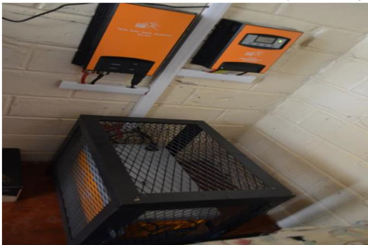
Figure 10. The battery box, inverter and controller of the SHS in one of the households at Watoto village
