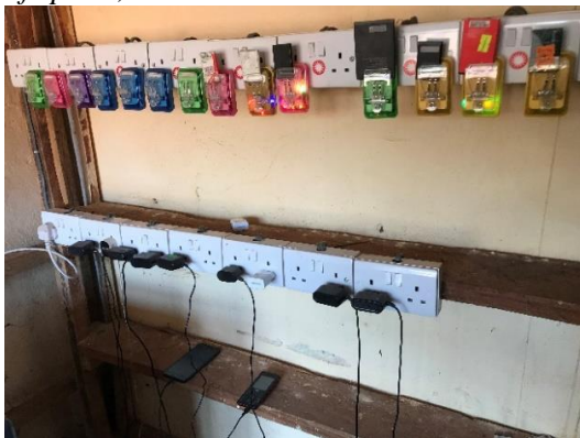
Figure 9. Kiosk for charging cell phones.
